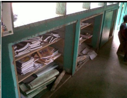
shelves need cabinet doors
