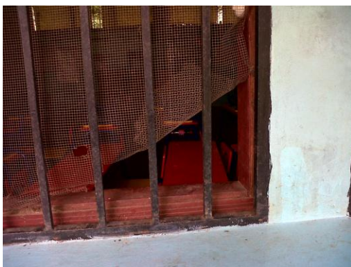
Screen windows need repaired
